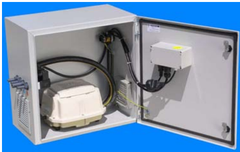
Picture 1 Indoor switch cabinet - interior view
