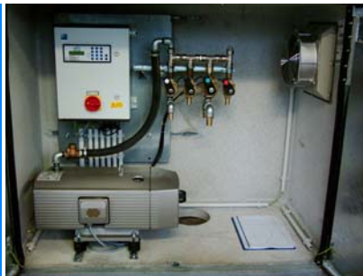
Picture 2 Two-door concrete cabinet - inside
